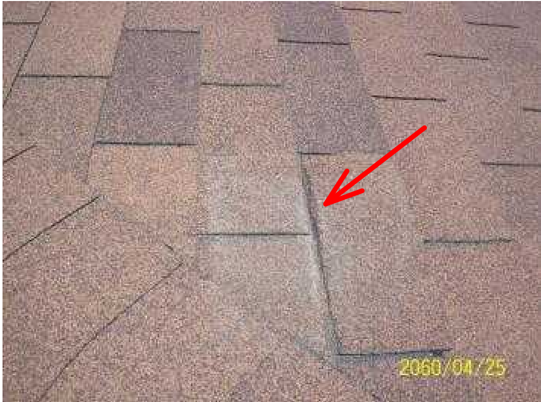
Fractured top of Tab.
