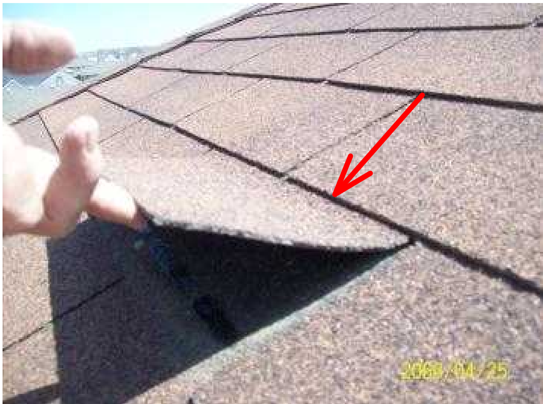
Example of the continouse effect of wind lifting tab,causing fracture.
