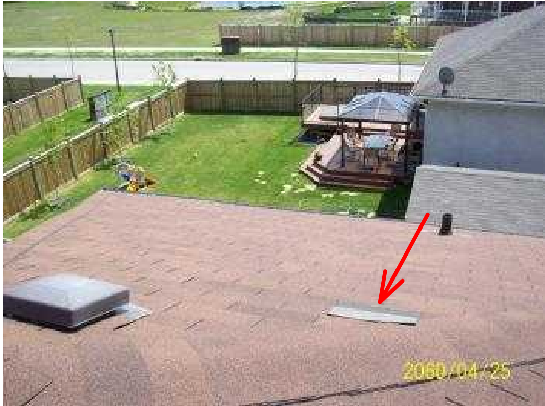
Wind blown shingle.
