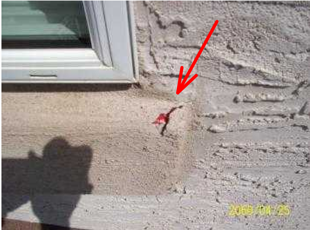
Damage to stucco
