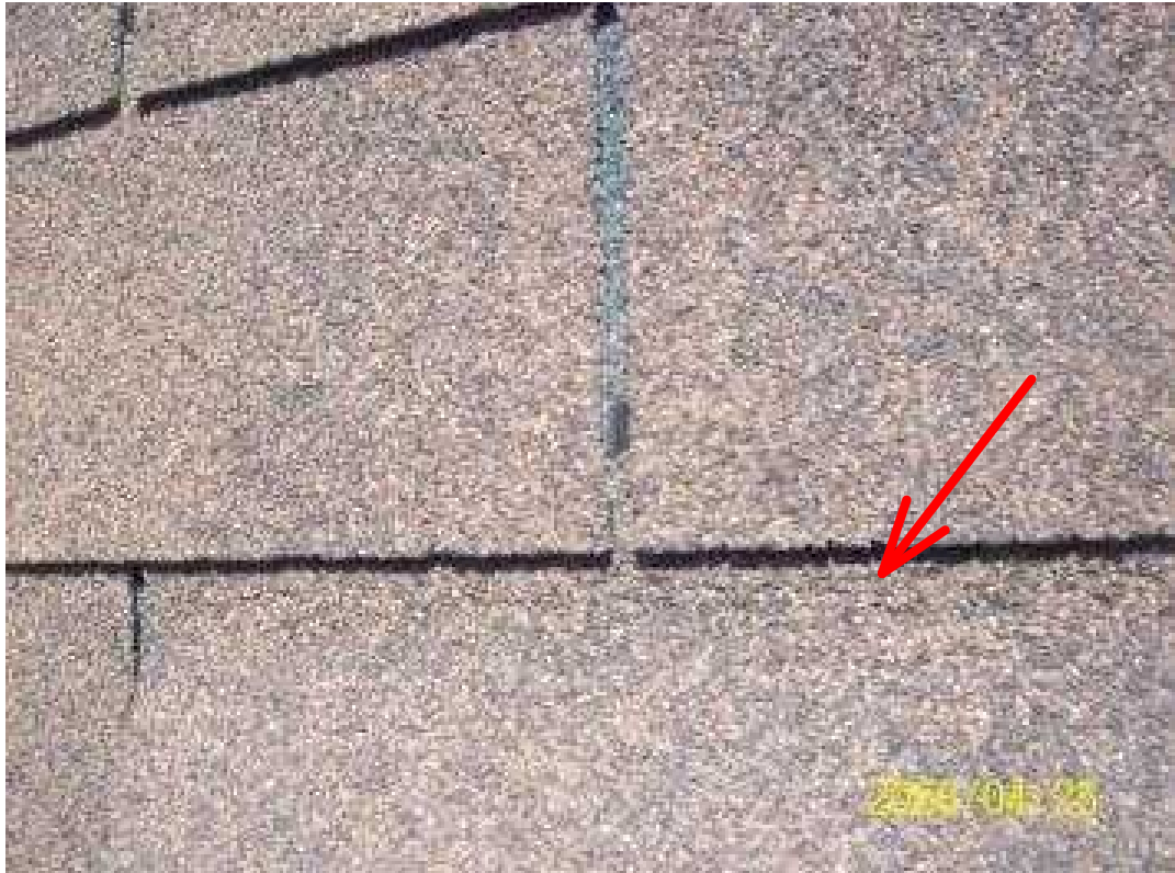
Fracture of the top of shingle tab. Due to wind lifting tab.
