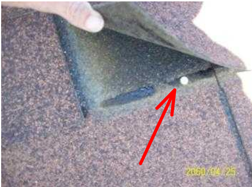
Contaminated Self sealing strip with dust.
