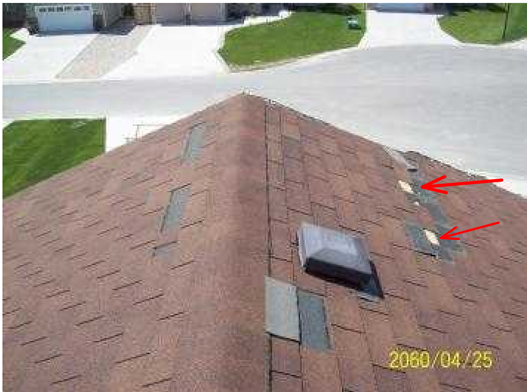
Windblown Shingles. Exposed plywood.
