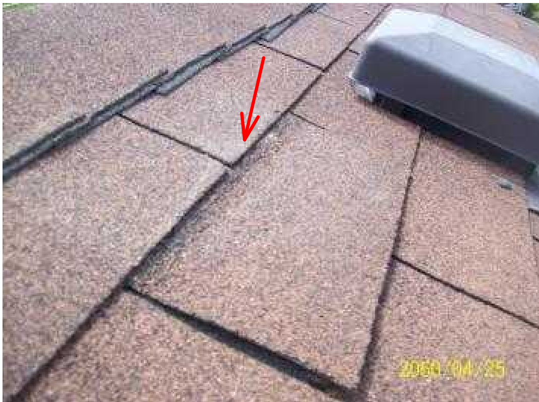
Damage to all slopes
